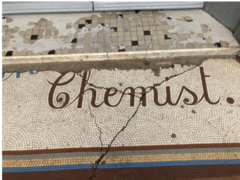
Figure 24: Damaged mosaic threshold at Broadway Mansions
