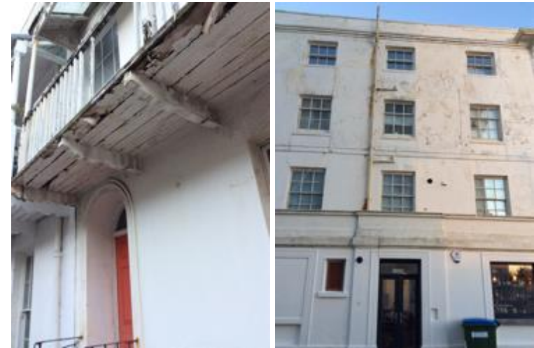
Figure 75: Examples of poorly maintained buildings on Warwick Road
